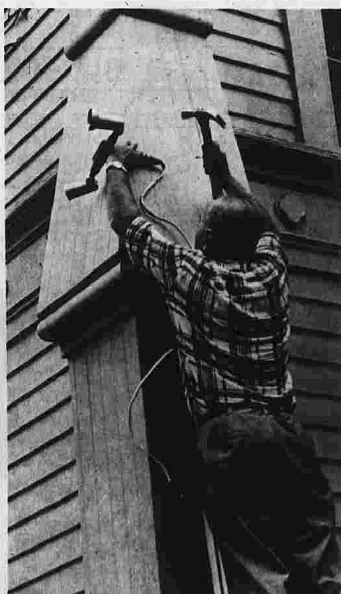
Outside lights are installed so the men can continue work after dark. Right, the refinished pews placed on new tile, are ready for a Saturday wedding, less than a week after the project began.
